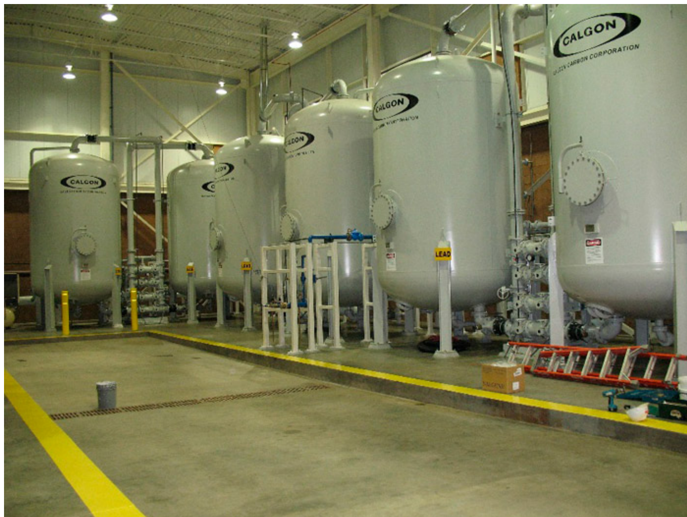
Figure 15-4. GAC treatment system, Oakdale, MN.
