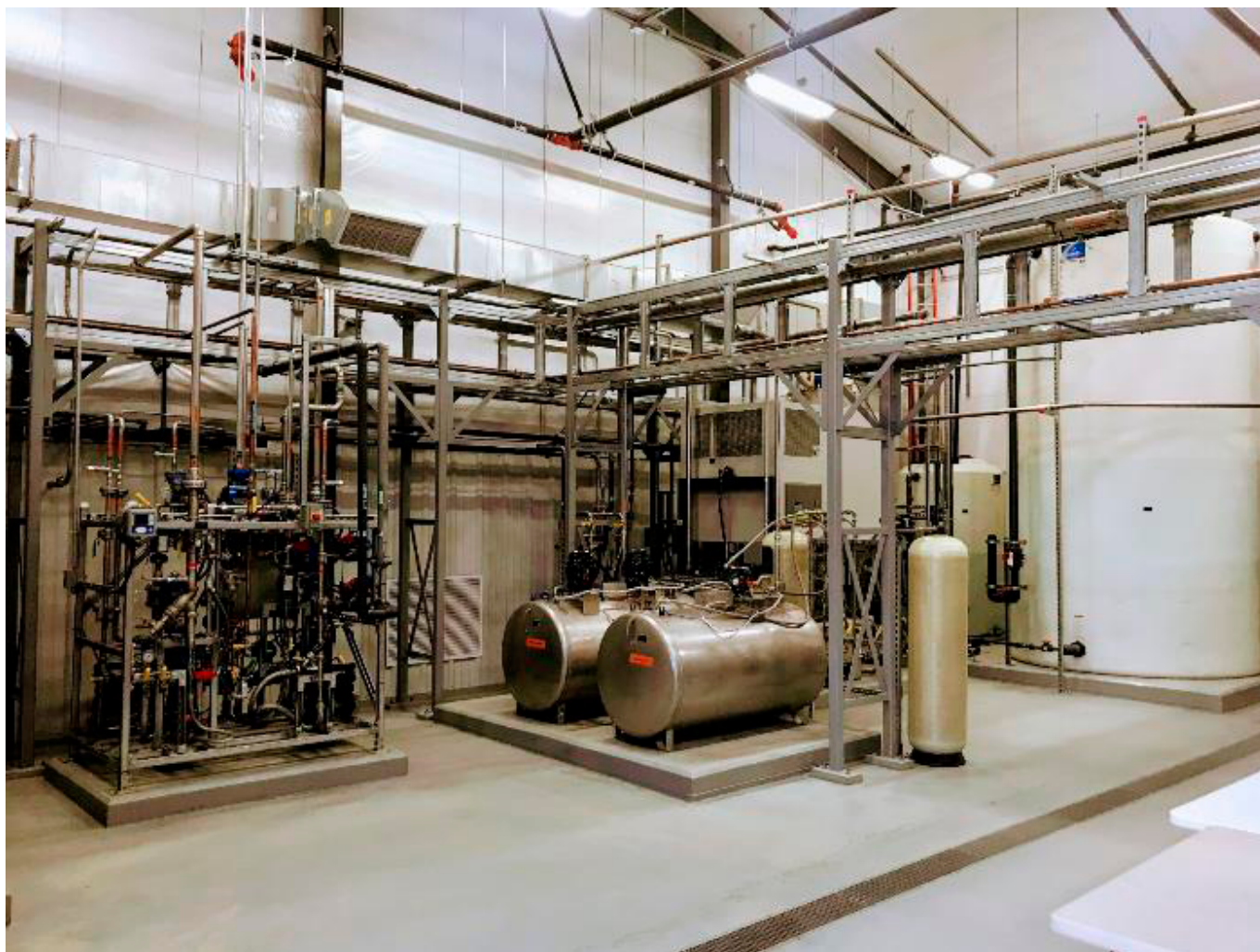
Figure 15-12. Resin regeneration system.
