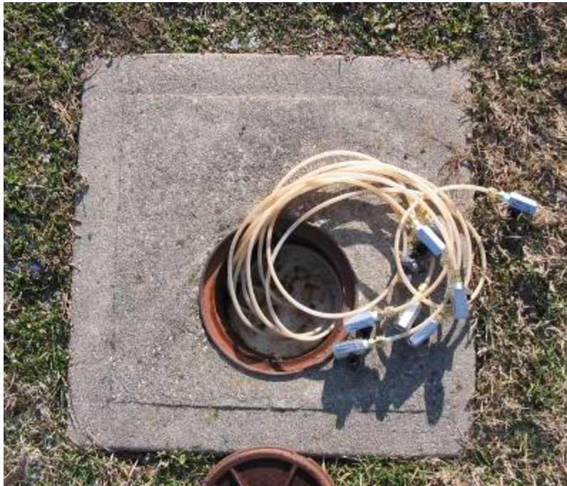
Figure G-7. Nested soil gas sample points in a single borehole (permanent probes with locking cap for repeated sampling).
