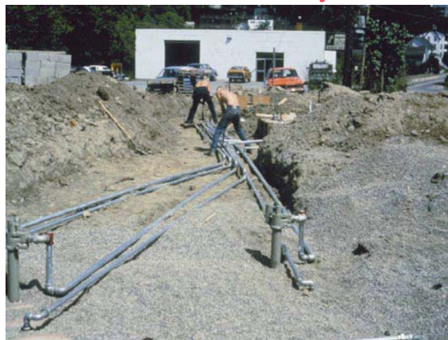
Galvanized-pipe installation from days of yore.
